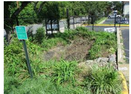
Bio-retention with signage
