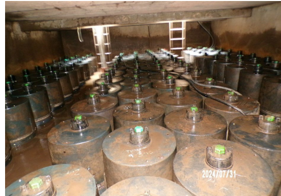
Before sediment/debris removed from structure
