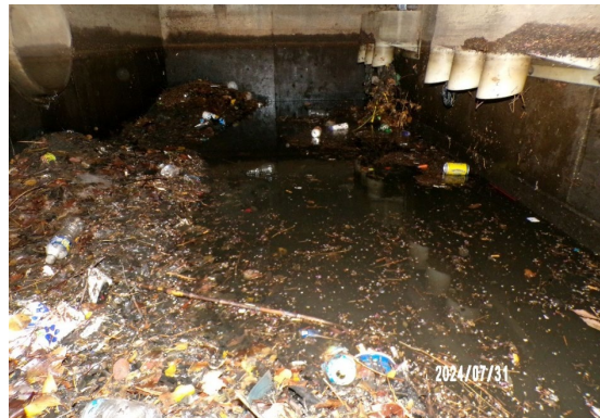
Before sediment/debris removed from structure
