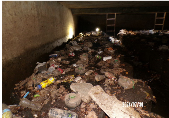
Before sediment/debris removed from structure
